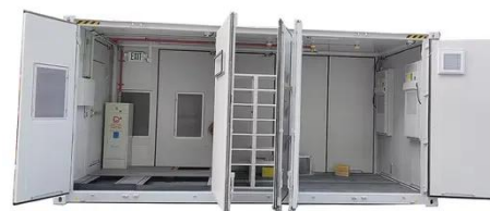
1075KW HH ESS
